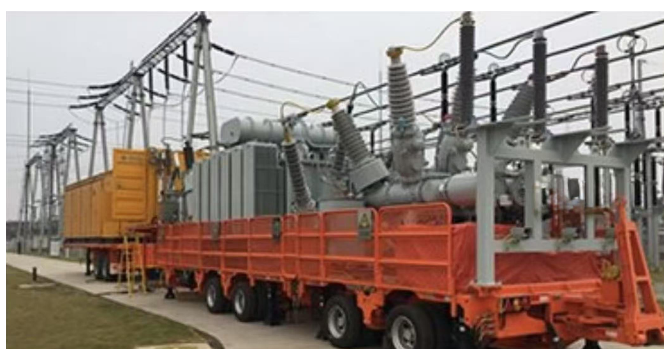
Mobile substation using traditional GIS
