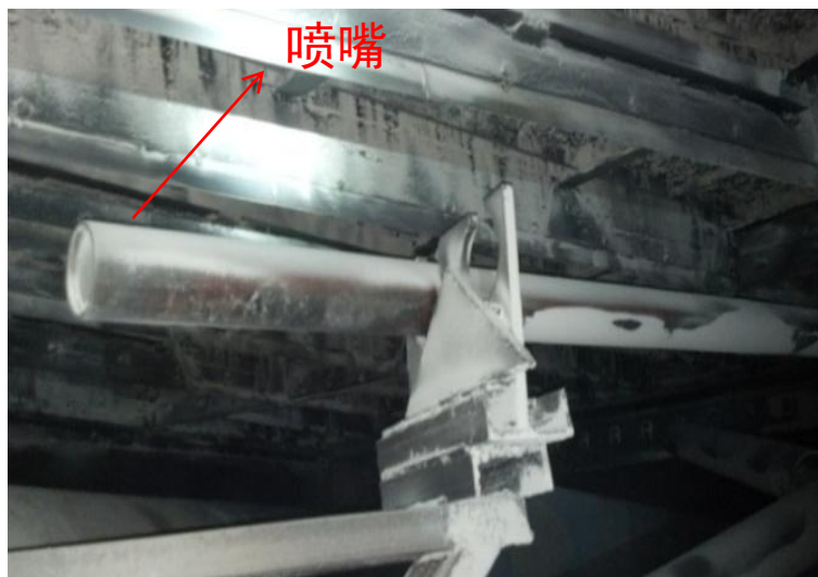
蒸气吹灰喷嘴偏斜
