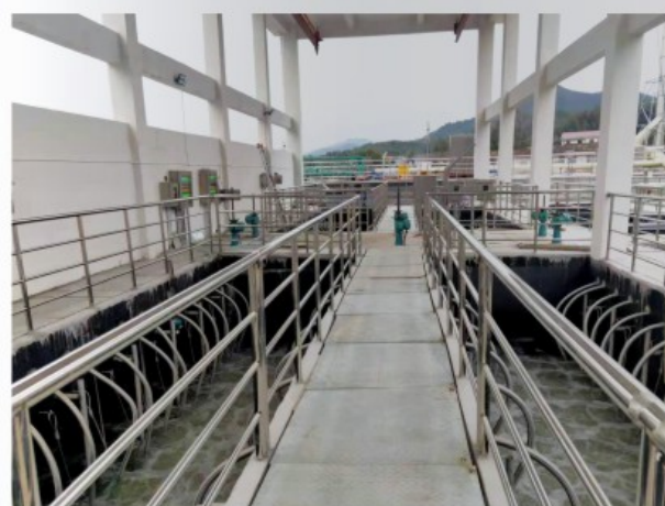
湖南省醴陵市横店产业园项目 Hengdian Industrial Park Project in Liling City, Hunan Province
