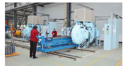
氢碎炉 Hydrogen decapitation furnace
