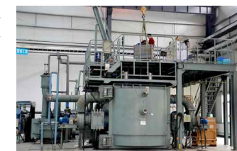
速凝薄带炉 Strip casting furnace
